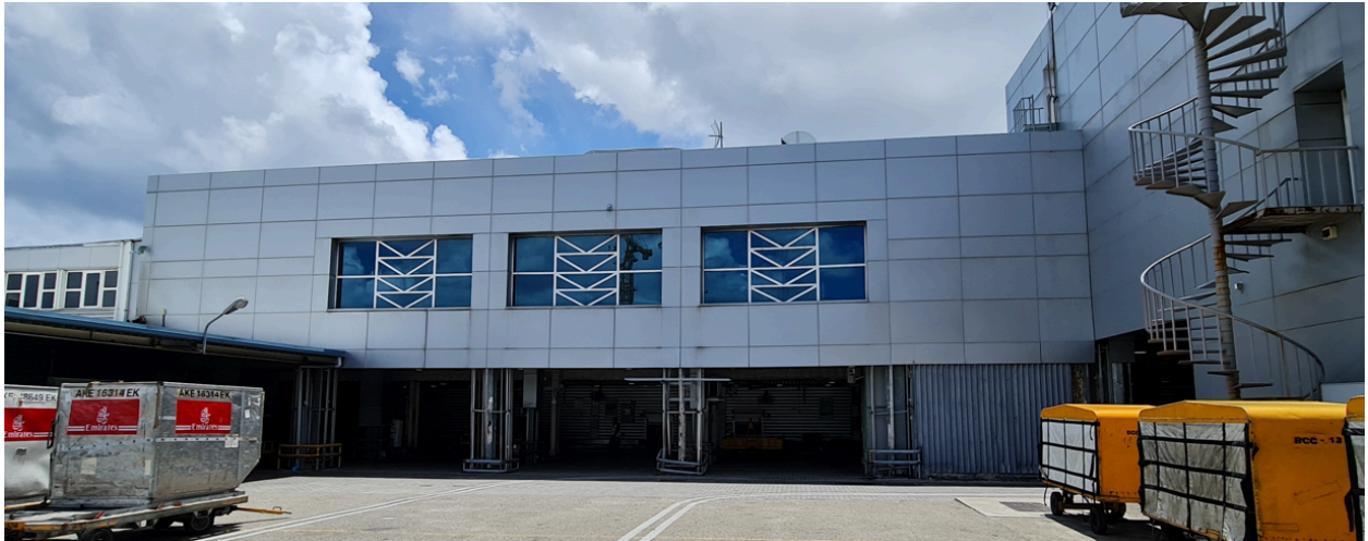
Structural conditions assessment of steel structure at Departure terminal extension building at Ibrahim Nasir International Airport (2022)
