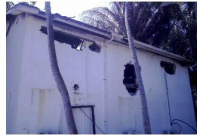
Existing structural conditions assessment of Fire damage of Store at Angsana Resort
