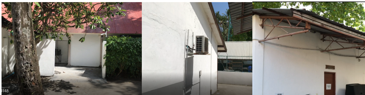
Existing structural conditions assessment and remedial action for, Main Kitchen, General Store & Housekeeping store of Clubmed Kanifinolhu (2021).
