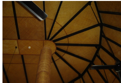
Existing structural conditions assessment of Rihiveli Restaurant of Angsana Resort.
