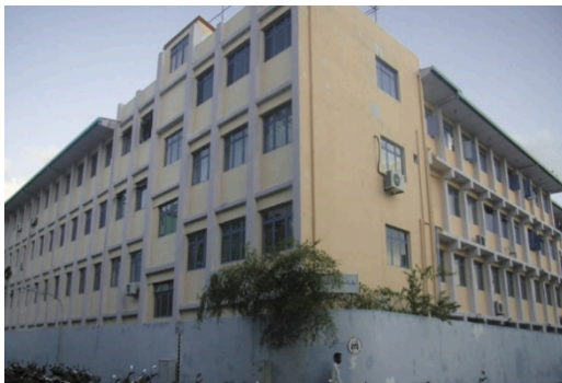
Existing structural conditions assessment and monitoring of Majeedhiyya school old building Monitoring during Holiday Inn Hotel Construction.
