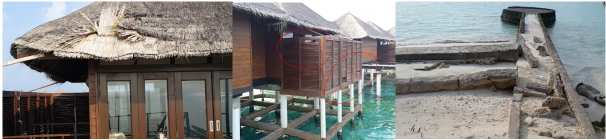
Weather damages to various structures at Coco Bodu Hithi Resort, for Sunland Hotels Pvt Ltd (2020)
